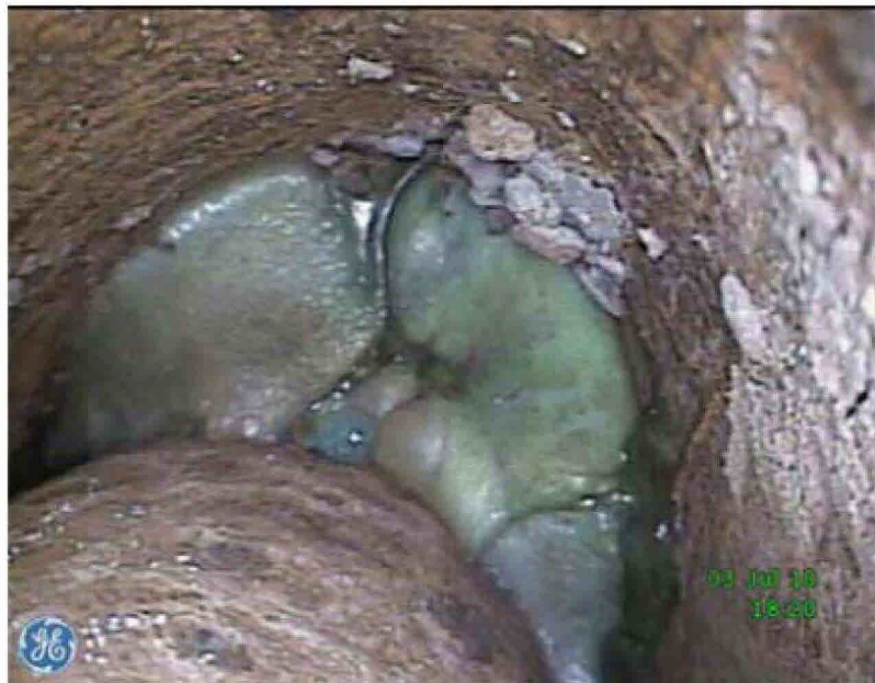
Figure 4 – Blockage in the kinked section of the riser 6
