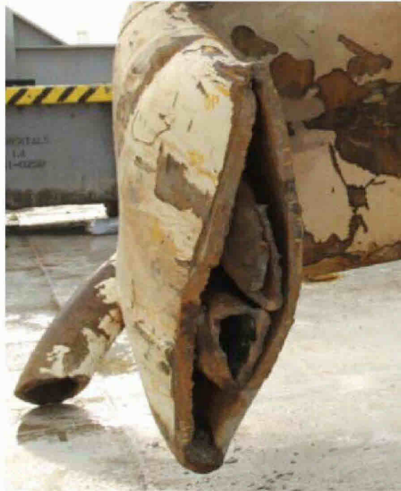
Figure 2 – Upstream section of the removed riser segment
