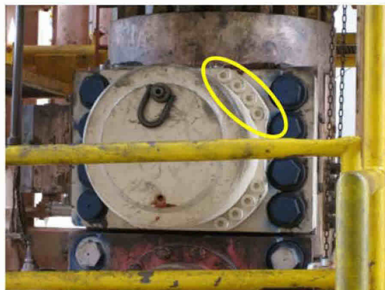
Figure 17.1 Casing shear ram operator bolts to be replaced.
