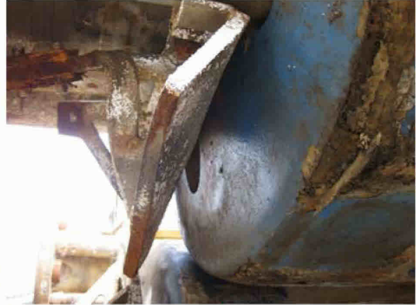
Figure 3: Damaged riser buoyancy thrust collar.
