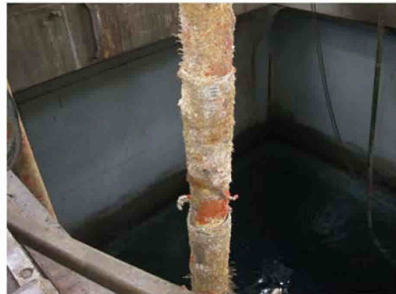
Figure 2: Damaged outer sheath on the moonpool hose.
