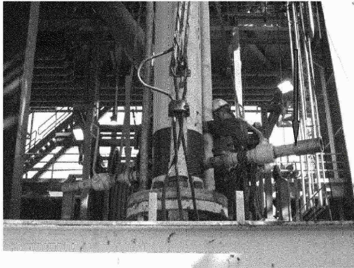
Figure 12.2: ROV operated ball valves (red arrows) installed and MUX cables installed on the riser joint.
