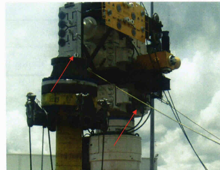
Pressure transducers and panel on 3-ram capping stack
