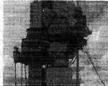
Pressure transducers and panel on 3-ram capping stack
