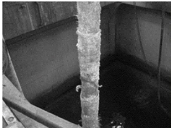
Figure 2: Damaged outer sheath on the moonpool hose.
