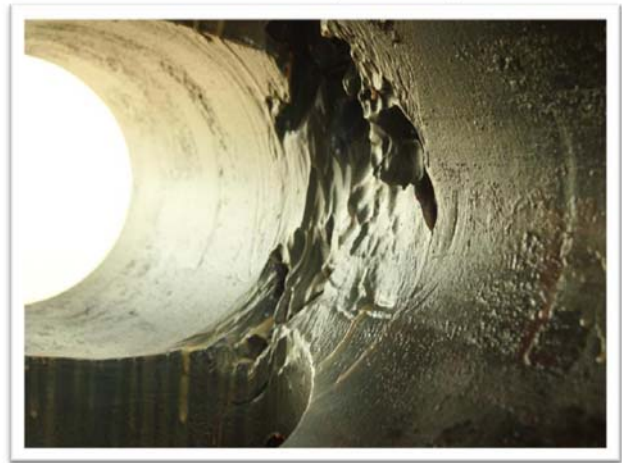
Well Bore (Erosion)
